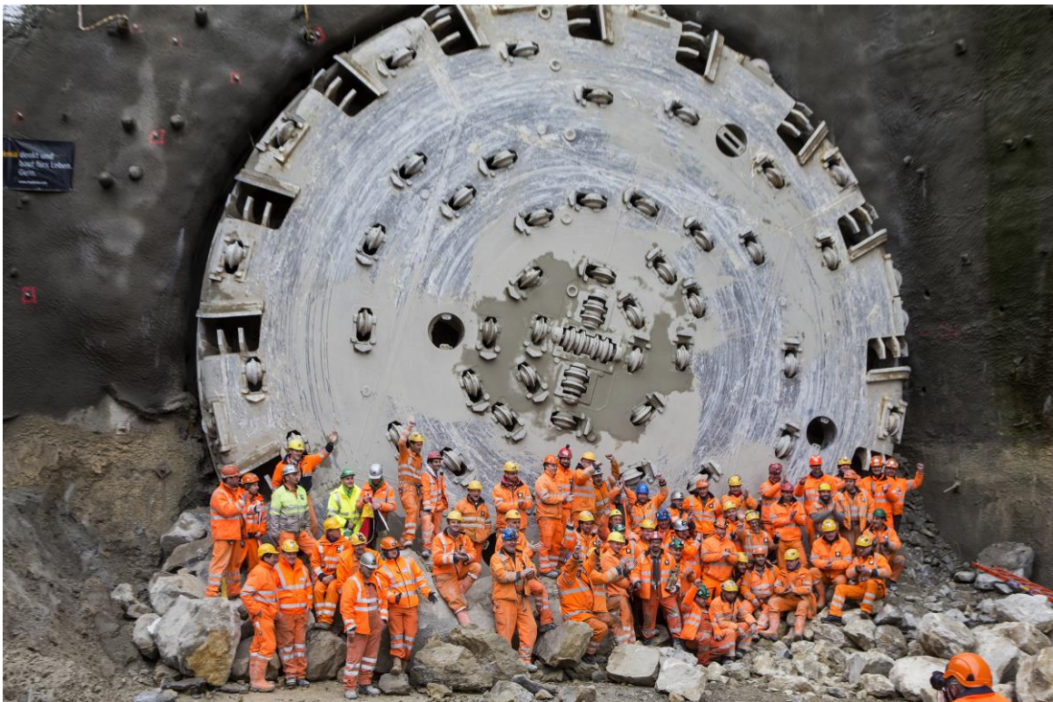
Historic moment: The Implenia team poses in front of the drill-head of the tunnel boring machine, which on 29 November 2017 broke through the last piece of rock, successfully completing the main drilling work on the Bözberg Tunnel (Photo: Keystone).
