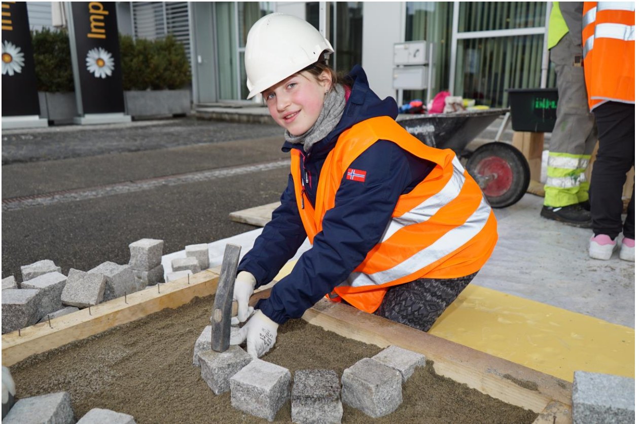
At Implenias National Futures Day, girls were given first-hand experience of the day-to-day work of masons and roadbuilders. (Source: Implenias)
