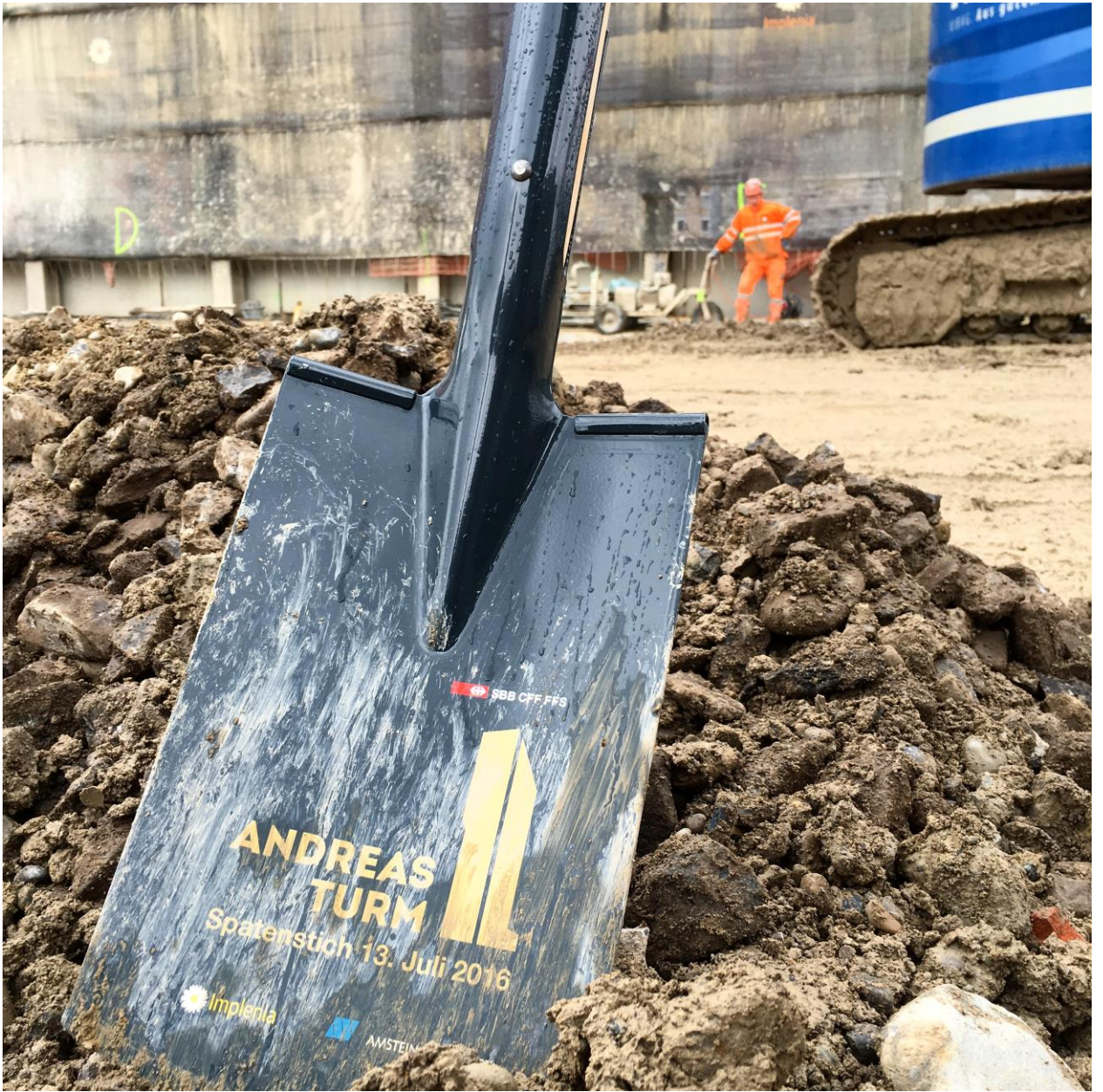
Let's wish for an accident-free construction period! Until May 2018 Implenia is realizing the 80-meter high-rise "Andreasturm" in Zurich-Oerlikon as total contractor. (Photo: Implenia)
