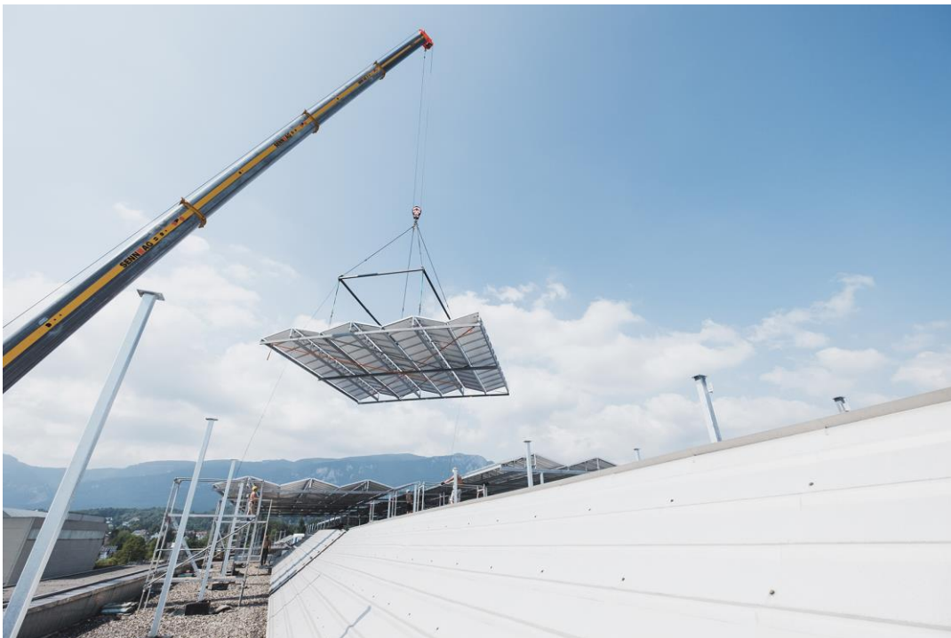
Building Switzerland's largest photovoltaic system, piece by piece: installing the system on the roof of Production Hall 330 at the Riverside industrial estate in Zuchwil. (Source: © SPS)
