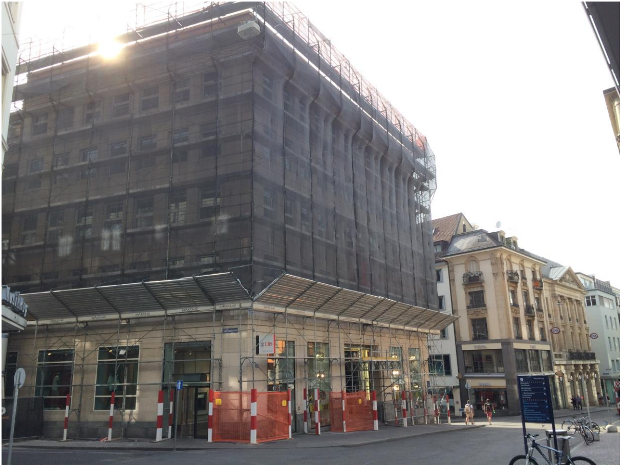
In the upper floors of the former bank premises, Implenía is building 143 hotel rooms for budget design hotel chain "Motel One". (Source: Implenía)
