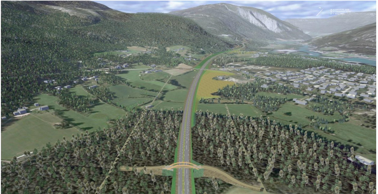
Around 80 kilometres northwest of Lillehammer, Implenía is building the new "E6", the largest single road infrastructure contract ever awarded by the Norwegian Public Roads Administration.
