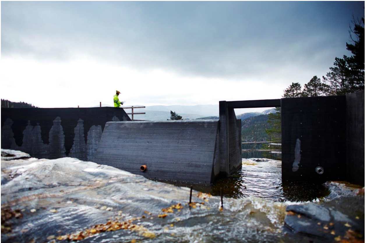
Construction of the new "Lysebotn II" hydro-electric power plant is another major order for Implenla in Norway.
