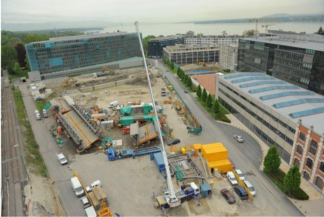
The building site of JTI's new international headquarters has opened on April 16, 2012. (Copyright : JTI)
