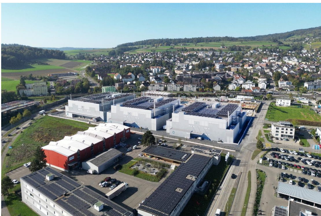
Implenia is building two more data centres for the Green Metro campus in Dielsdorf near Zurich (image: © zvg. bfarchitekten.ch).
