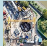
Heating tunnel, Hamburg, Germany
