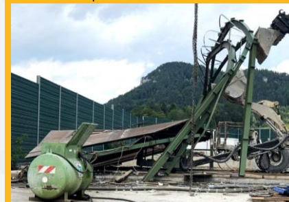
After the collapse
