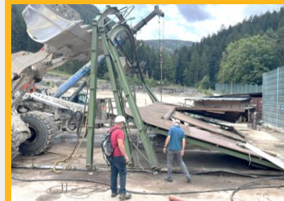
After the collapse
