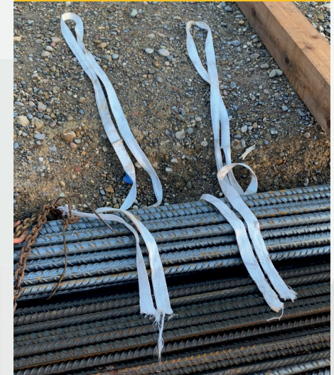
Disposable lifting slings involved in the accident.
