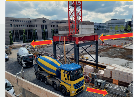
Construction site organised in such a way that reversing is unnecessary; here, for example, for the delivery of concrete.
